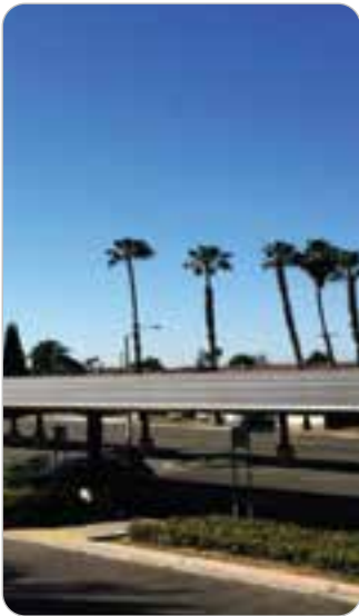
School Project USA | 3.3MW | 2013
