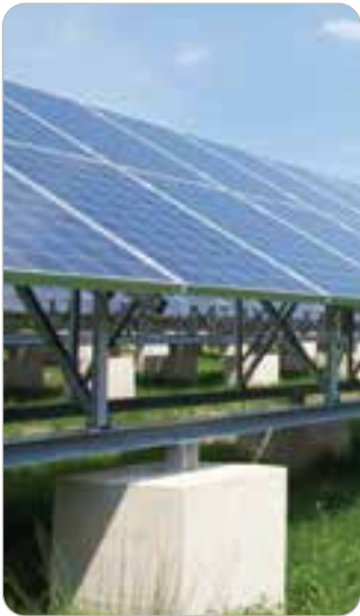
Alps Project Germany | 1.5MW | 2010
