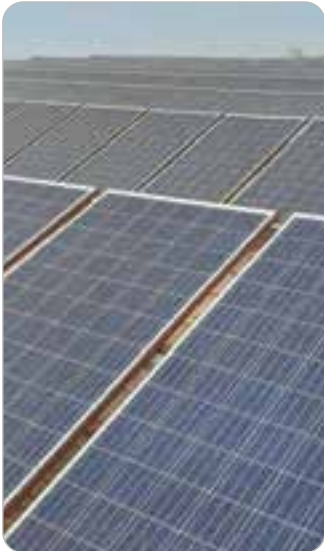
Yemen Project Yemen | 1.0MW | 2019
