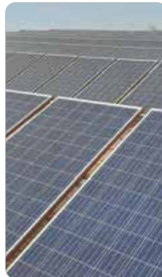
Yemen Project Yemen | 1.0MW | 2019
