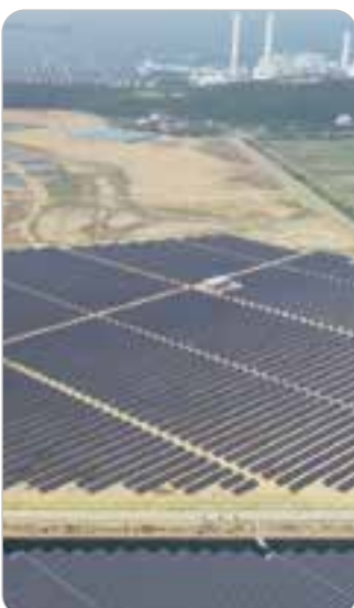
Dangjin Project Korea | 25MW | 2020
