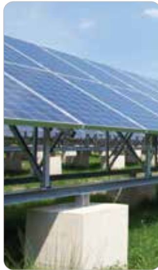
Alps Project Germany | 1.5MW | 2010
