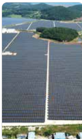
Samyang Project Korea | 17MW | 2020
